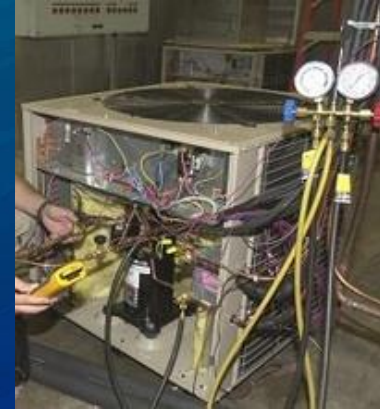
High Efficiency HVAC Systems and Controls
