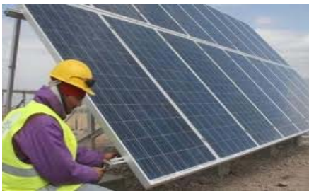
In April 2011, the Province of San Juan commissioned the solar farm San Juan I. This pilot installation located in Ullum has an installed capacity of 1.2MW.
