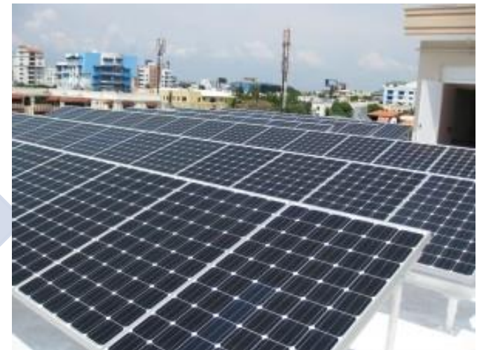
PV System National Energy Commission (Dominican Republic) Co-financed by CREDP/GIZ
