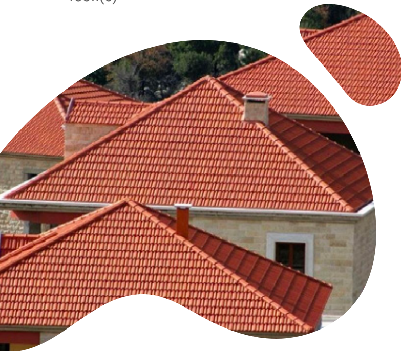
Figure 2 Hipped Roof design. Hipped roofs are better suited to withstand the strong winds associated with a tropical cyclone. Source: art-profy.com
