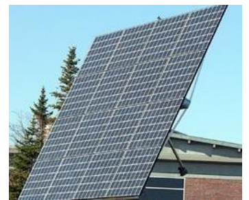
Photovoltaic panel for a school
