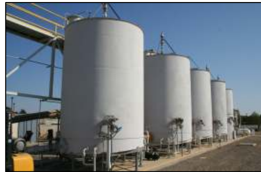
Anaerobic Sequence Batch Reactor (ASBR)
