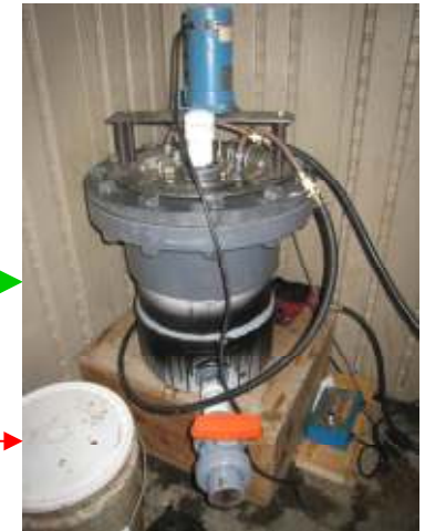
CSTR anaerobic digester
